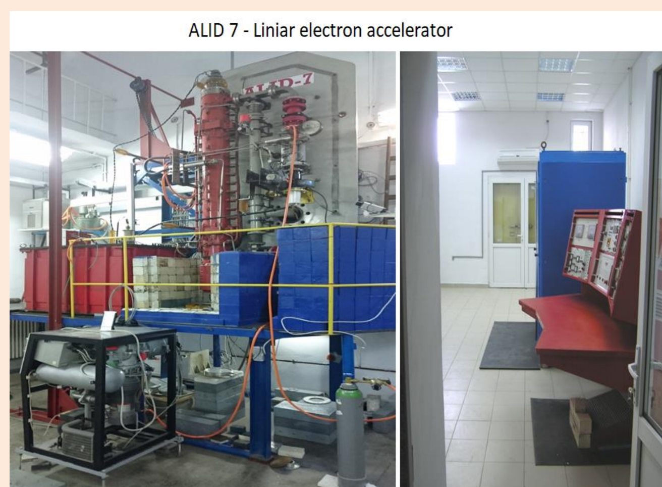
Figure 1. ALID 7 linear electron accelerator: Irradiation installation and control desk
